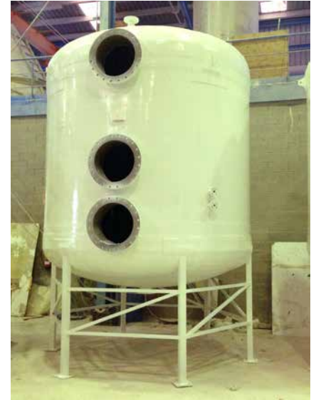
Filters tank Vertical sand
